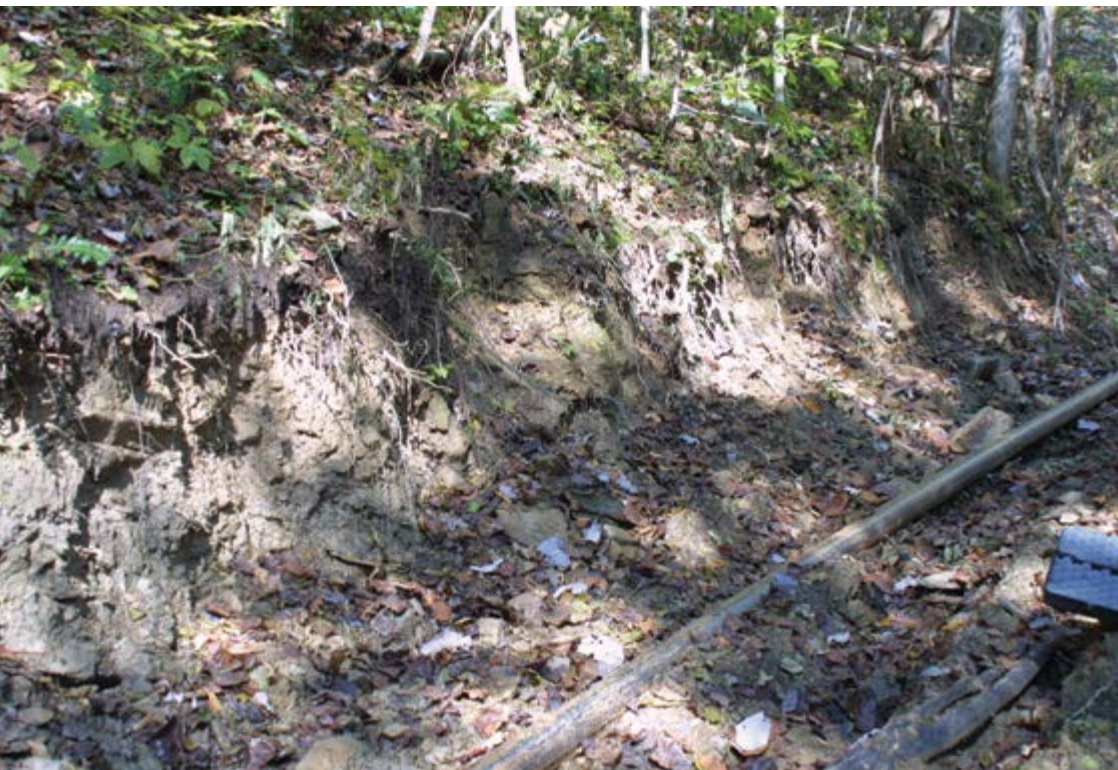
Below: Figure 2. Goldenseal ( Hydrastis canadensis ) population destroyed by gas line construction in southern West Virginia. Photo © Dean Myles 2004
